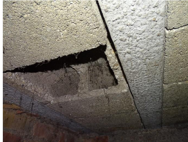
Abb. 8: Offener Hohlblockstein in Kellerdecke
